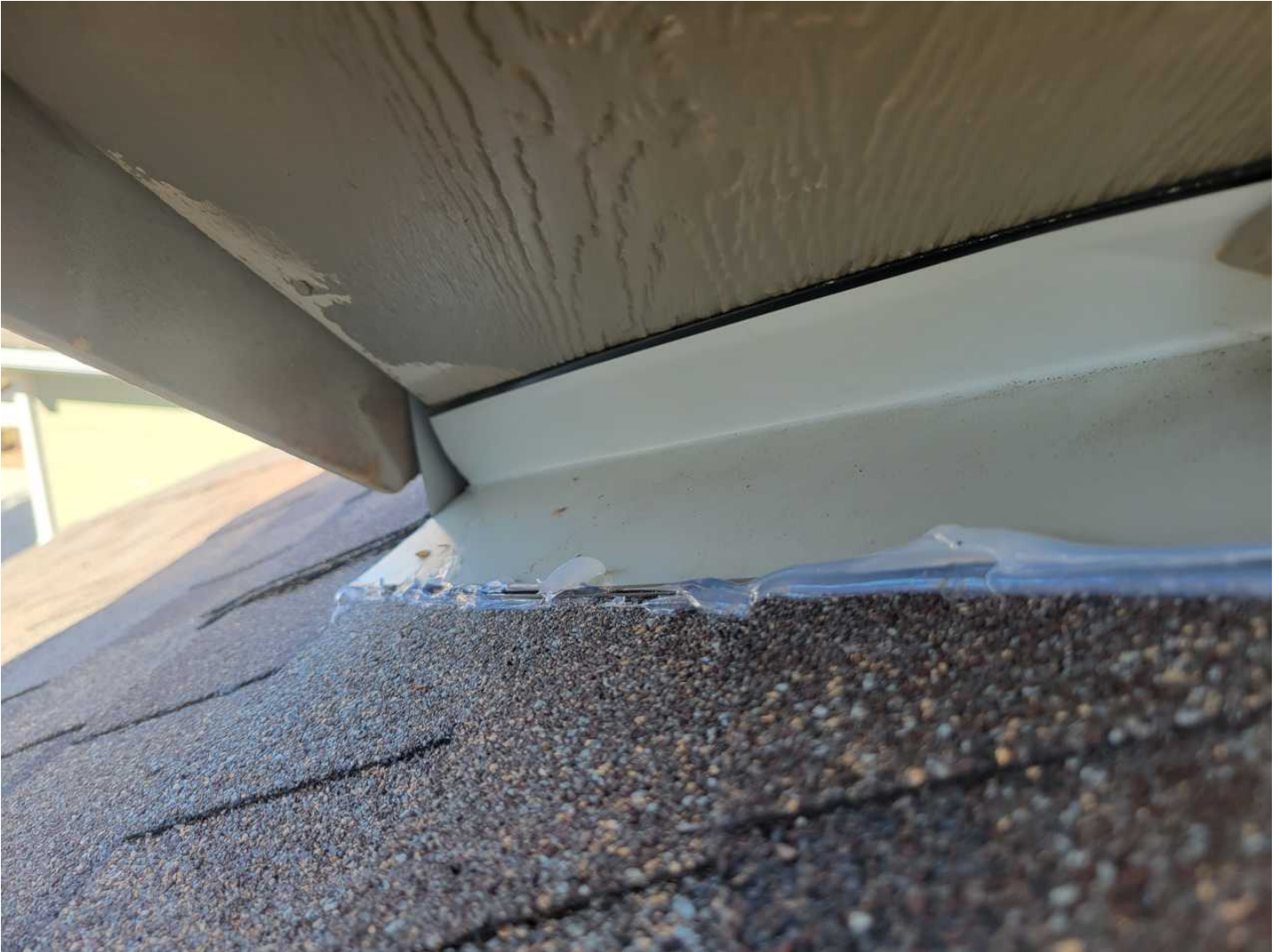
23 24-silicone and flashing under soffite vent as e
